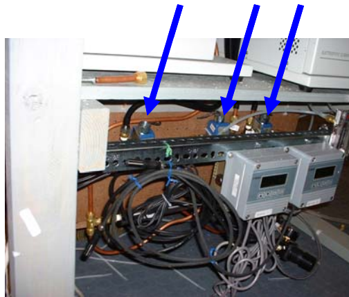
Arrows Point to Electrically Actuated Solenoid Valves Used in Sheath Drying Loops for NDMA and LDMA. Valves are partially obscured by support for Vaisala RH Meter Electronics
