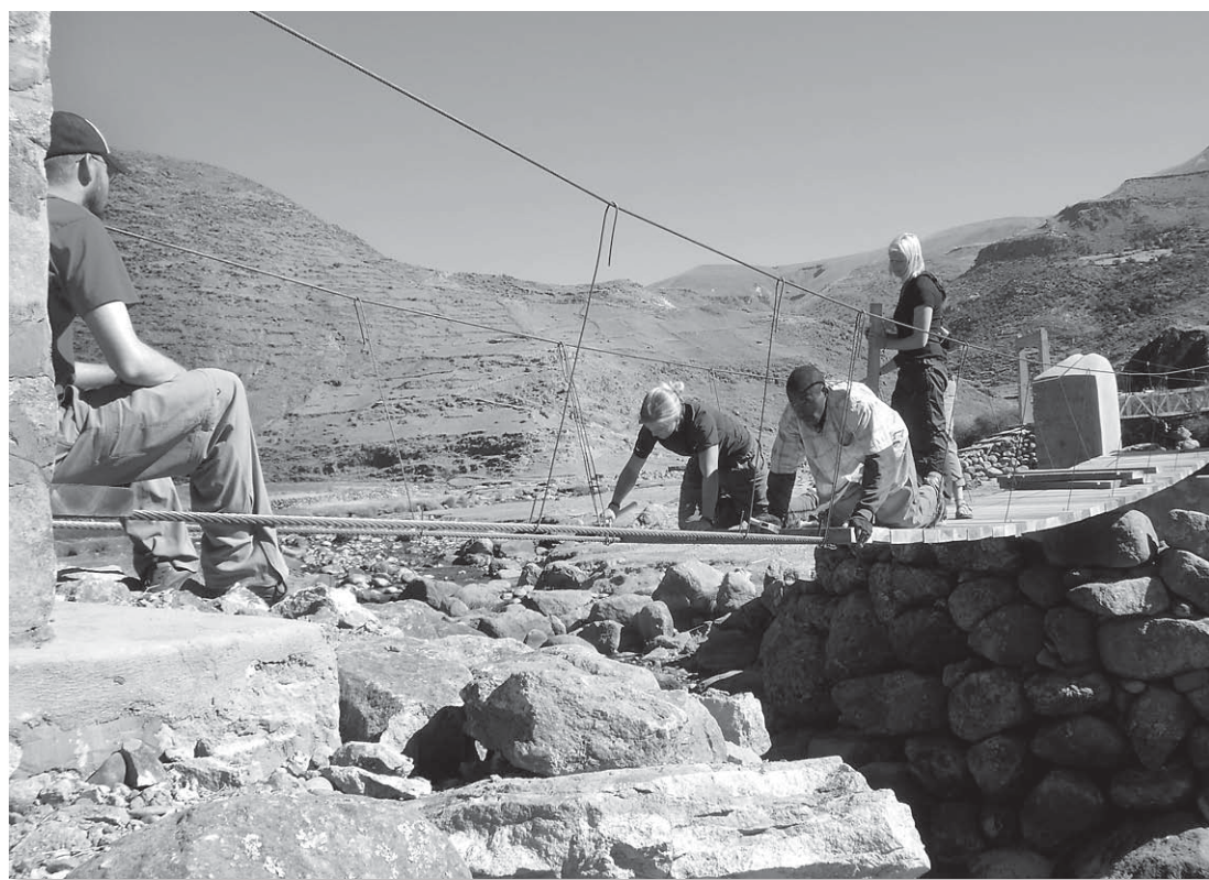
Members of Continental Crossings lay planks across the cables of the new pedestrian bridge near Yavina, Peru.
